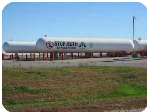
Figure 10.15.1: An ammonia storage tank.
