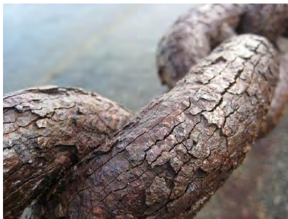
Figure 3.5.2: Heavy rust on the links of a chain near the Golden Gate Bridge in San Francisco; it was continuously exposed to moisture and salt spray, causing surface breakdown, cracking, and flaking of the metal. (CC BY-SA 3.0; Marlith).
