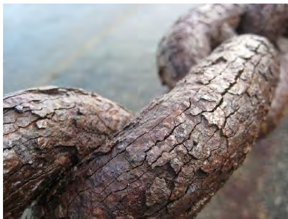
Figure 3.5.2: Heavy rust on the links of a chain near the Golden Gate Bridge in San Francisco; it was continuously exposed to moisture and salt spray, causing surface breakdown, cracking, and flaking of the metal. (CC BY-SA 3.0; Marlith).
