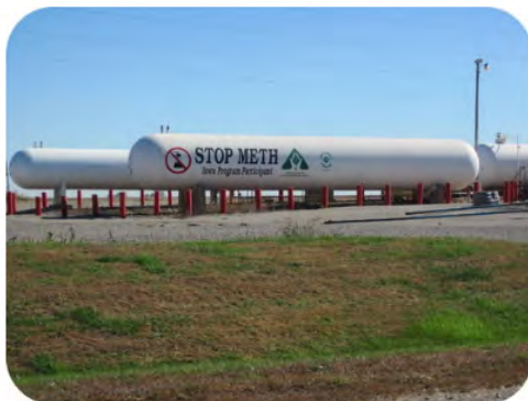
Figure 10.15.1: An ammonia storage tank.
